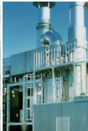
Example installation of Deodorizing equipment
